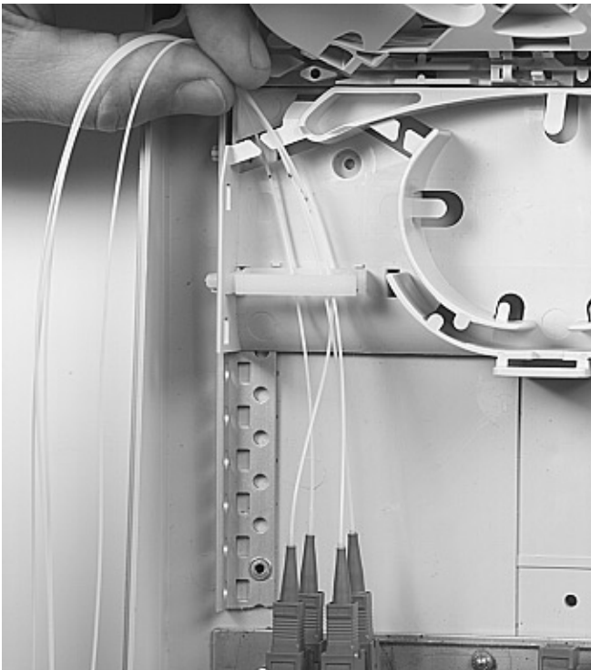
5.1.4 Mount the pigtail connectors in the adapters and route the pigtails to the splicing trays.
