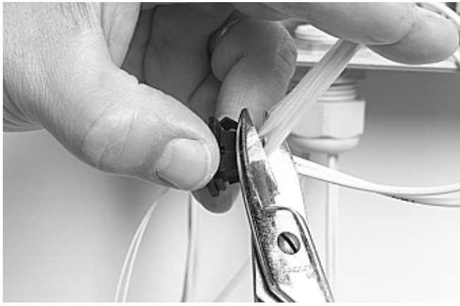
5.2.8 Cut the Kevlar yarns at the connector and install in the patch panel adapter.
